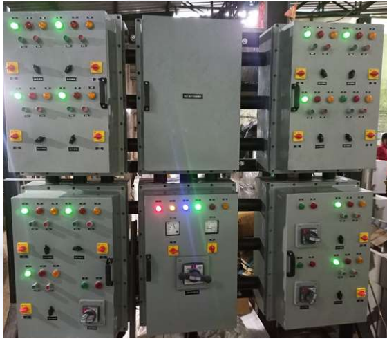
MOTOR CONTROL CENTER (MCC)
